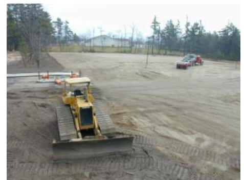
The Boat Company Parking Lot on the Donegal Bay Road under construction in mid-November.
